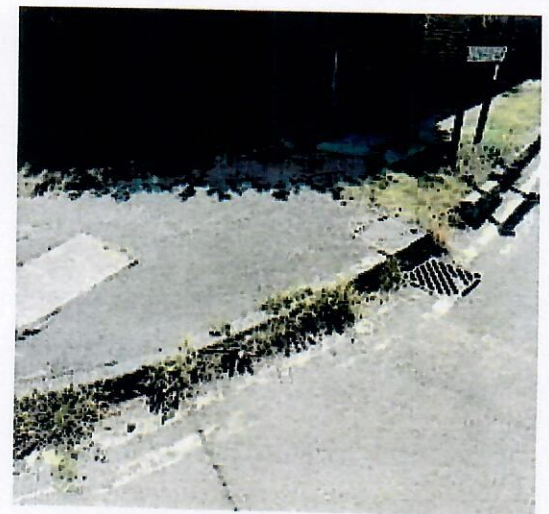
Weeds and vegetation Queensway and Fyfield Road obscuring important road sign warning drivers of a school
